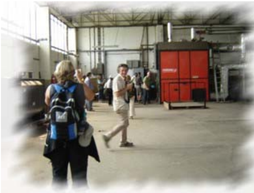
Figure 11: Inspecting a Wood Chip Burner in Kaltensundheim.
